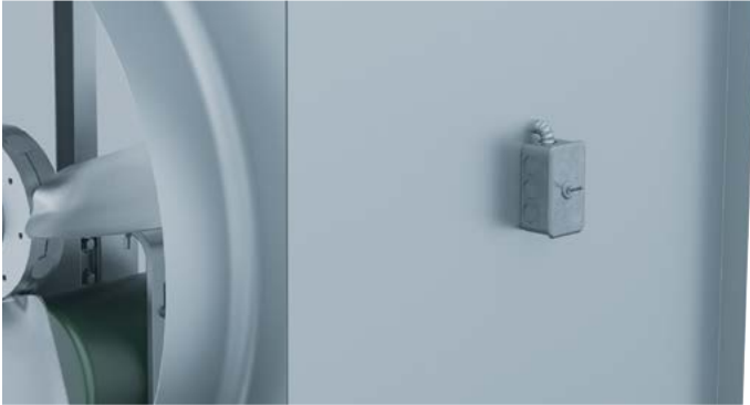
NEMA 1 Disconnect Switch
