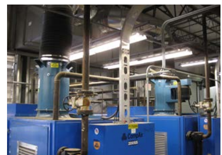
Air Compressor Heat Exhaust Fans
