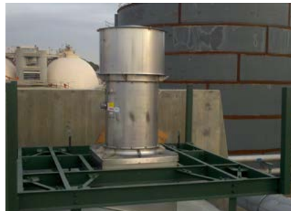
Exhaust for Digester Gas Compressor Facility
