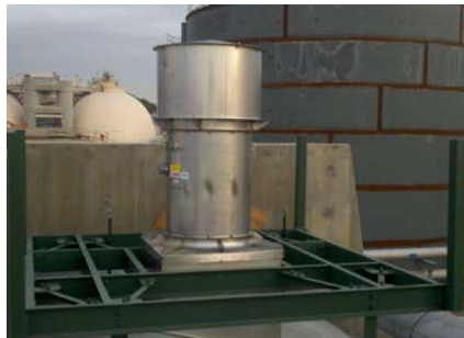
Exhaust for Digester Gas Compressor Facility
