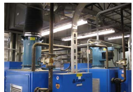
Air Compressor Heat Exhaust Fans
