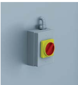
NEMA 4 Disconnect Switch
